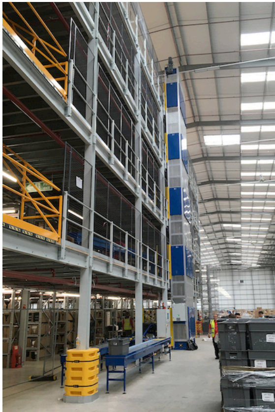
One of two lifts supplied by Nerak to Missguided's new warehouse in Trafford Park, Manchester
