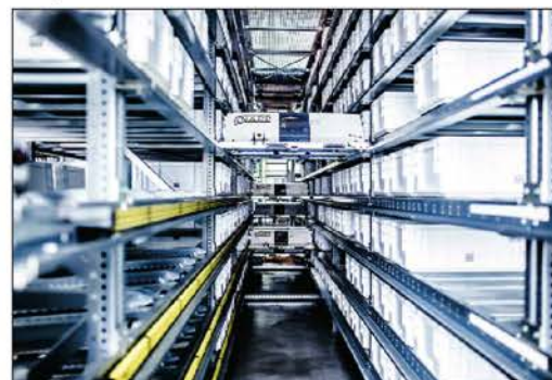
With the OSR Shuttle™, every article in storage is ready for picking - ©KNAPP.
