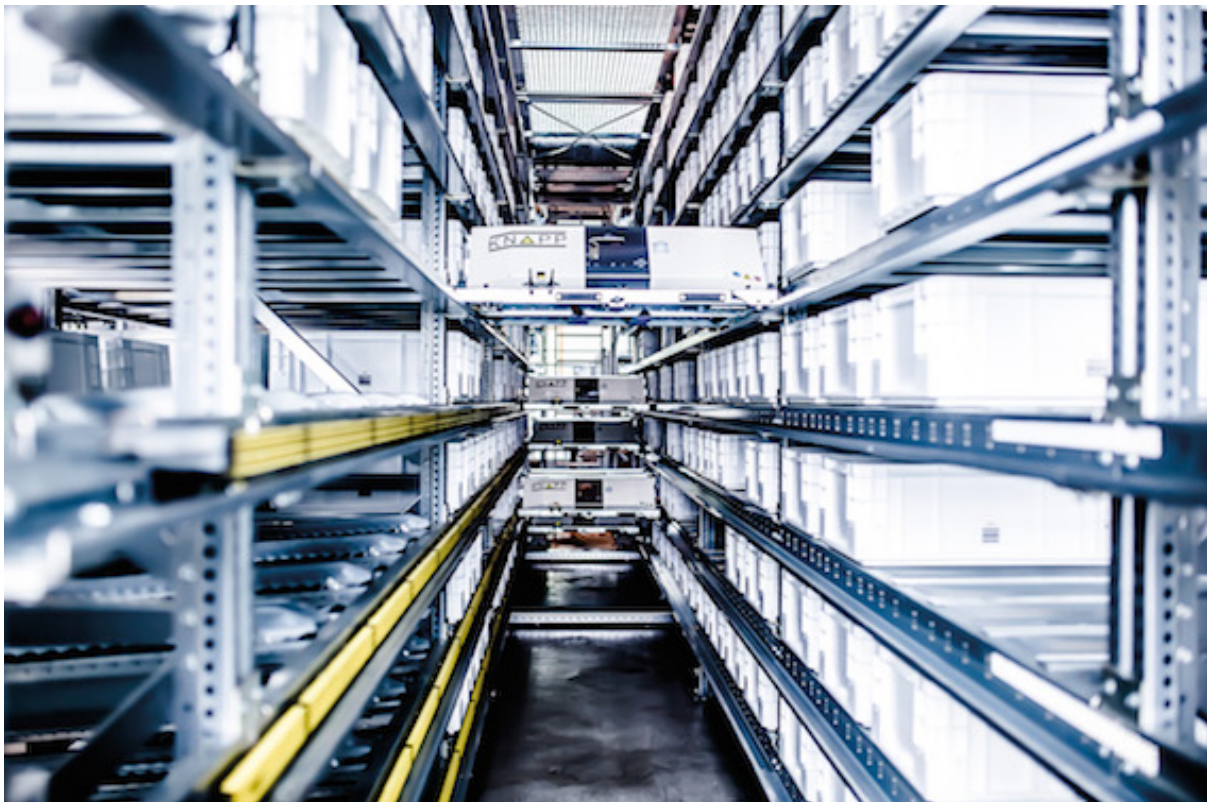
With the OSR Shuttle™, every article in storage is ready for picking – ©KNAPP
